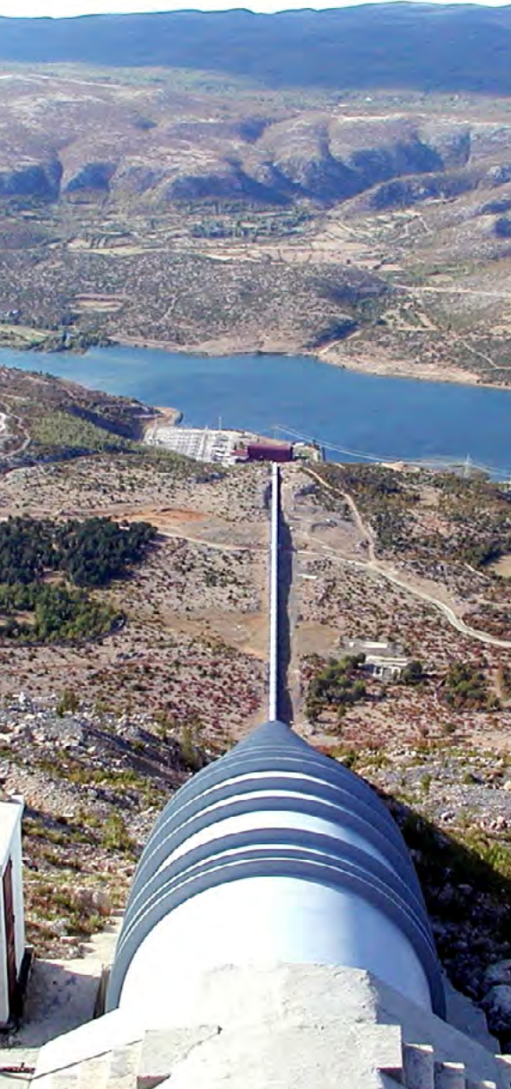
HPP Velebit, hydro pumped power station.
